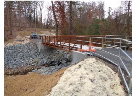
The section of the Tanyard Branch Trail that connects McMaster and Jay Streets is now complete. We have started on design of the final phase that will continue the trail to Umstead Park.
