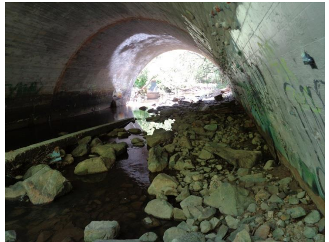
The project will take advantage of the existing culvert that takes Bolin Creek under Martin Luther King Jr. Blvd.
