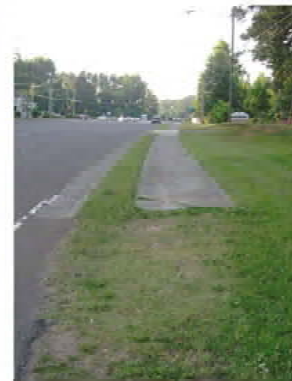
SIDEWALK LACKING PAVED CONNECTION NEAR HOMESTEAD ROAD
