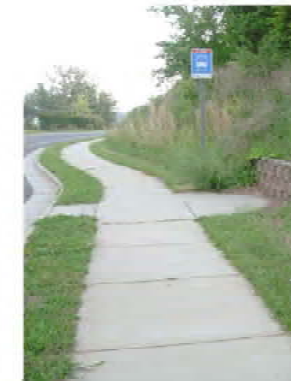
BUS STOP WITHOUT BENCH NEAR WESTMINISTER DRIVE
