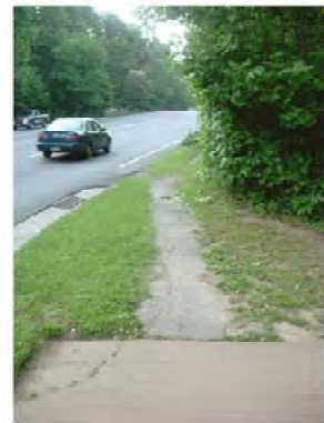
WORN FOOTPATH NEAR BUS STOP AT TIMBER HOLLOW APARTMENTS
