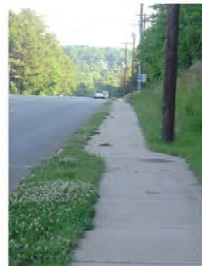
IRREGULARLY ORIENTED SIDEWALK
