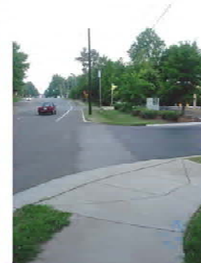
SIDEWALK LACKING PAVED CONNECTION NEAR NORTHFIELD DRIVE
