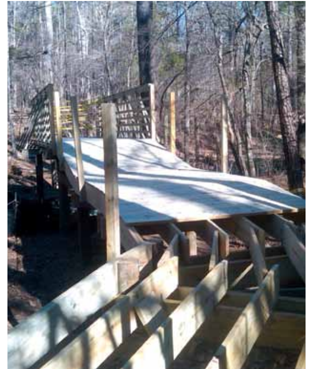
Bolin Creek Bridge Top and bottom right: under construction Bottom left: completed
