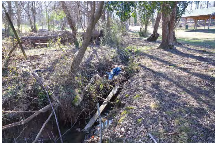
Area 7 View of Head Cut Facing Upstream
