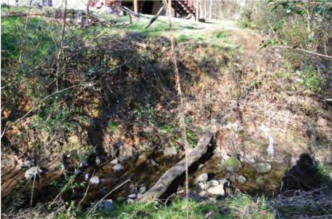
Erosion on private property to the north – pre-construction
