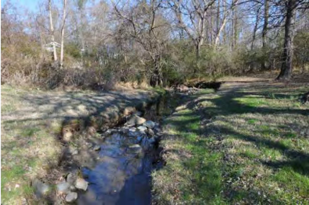
Erosion on the west channel in Baldwin Park – pre-construction
