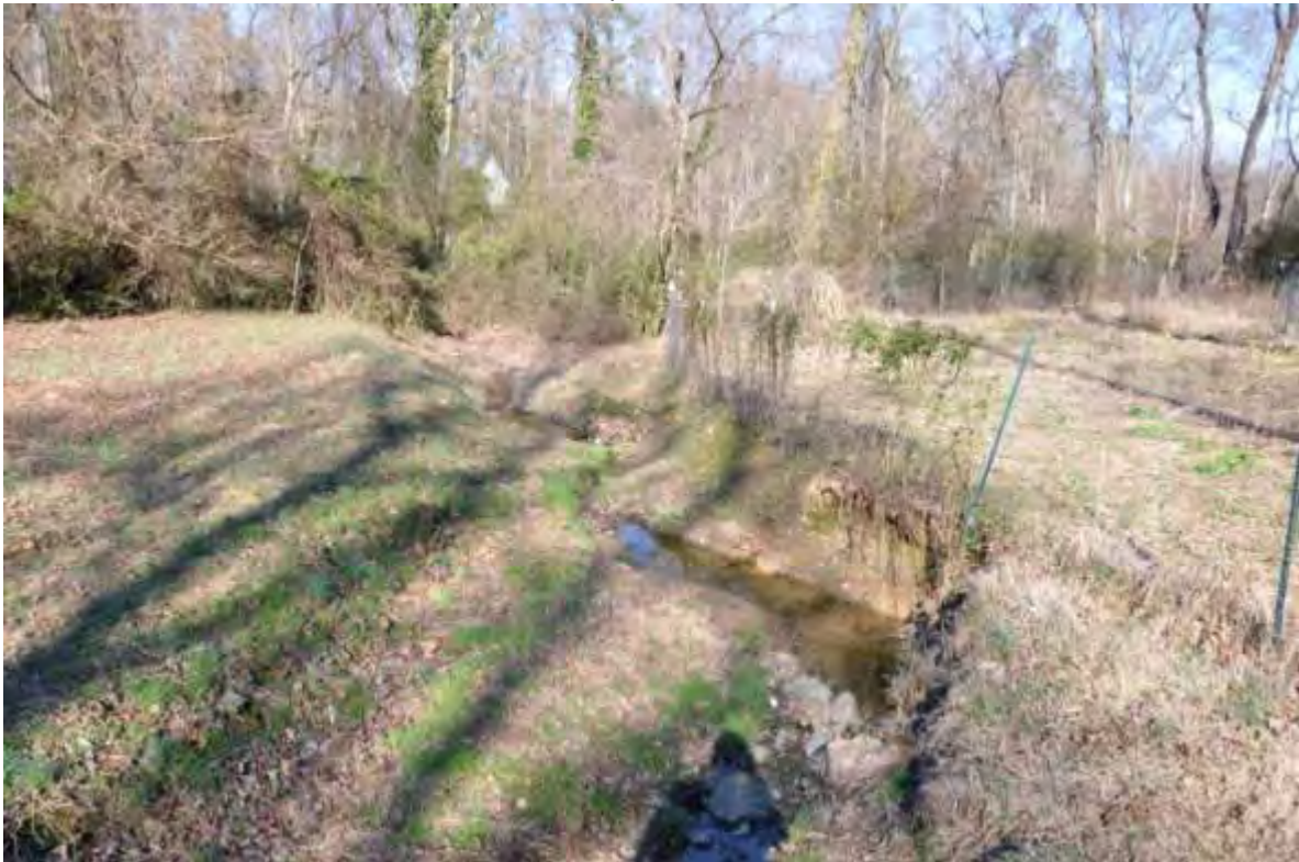
Erosion on the east channel – pre-construction
