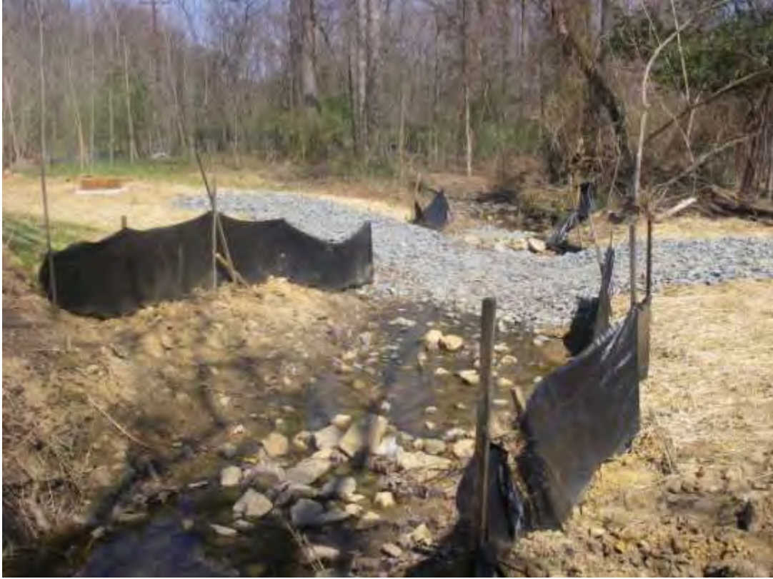
The OWASA crossing done incorrectly
