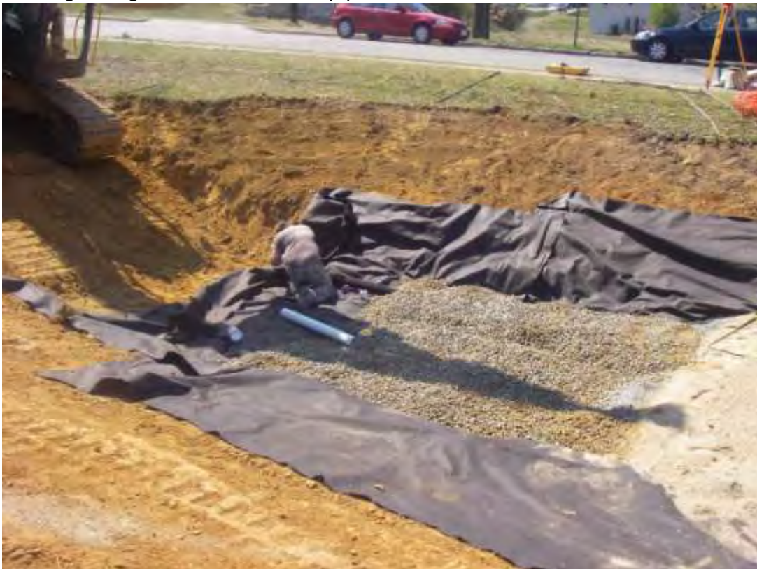
Laying the filter fabric and hooking up the pipes in the bioretention
