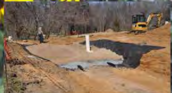
During construction: lined with geotextile fabric, added a gravel layer with underdrains, and several feet of high infiltration soil
