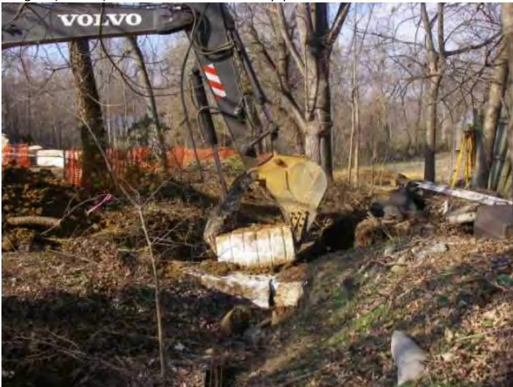
Placement of the giant rocks perpendicular to the channel to create the step-pools
