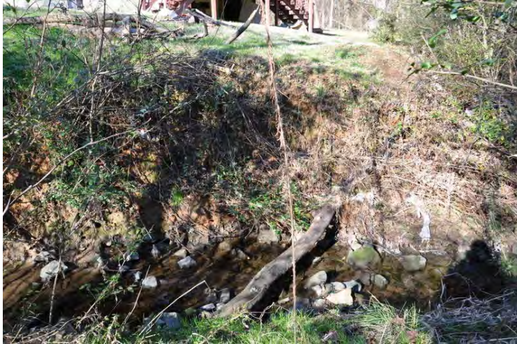
Area 3 Eroding Streambank
