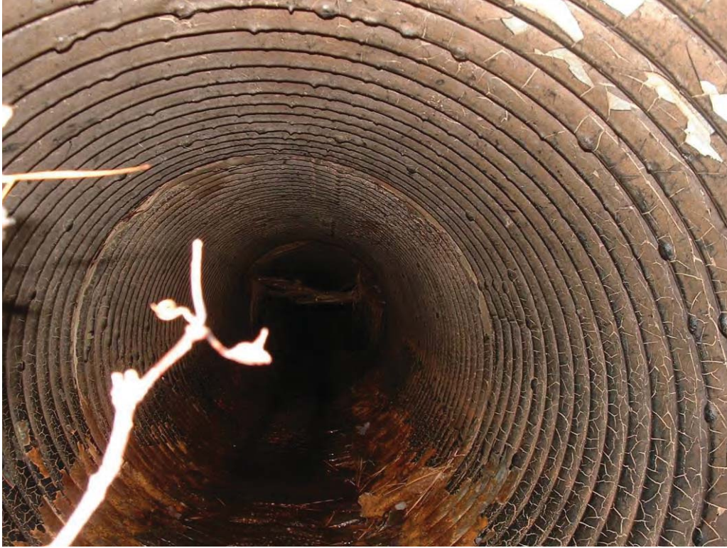
deterioration in culvert
