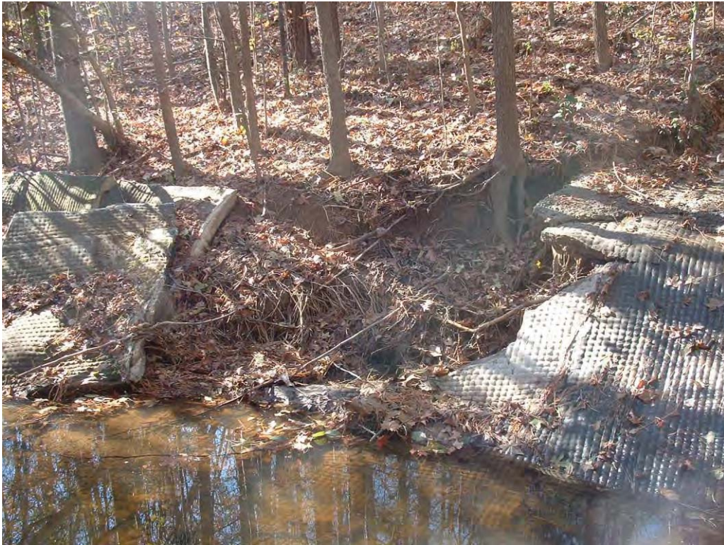
Exhibit C-5. Photos of Failing Sections of Channel Lining
