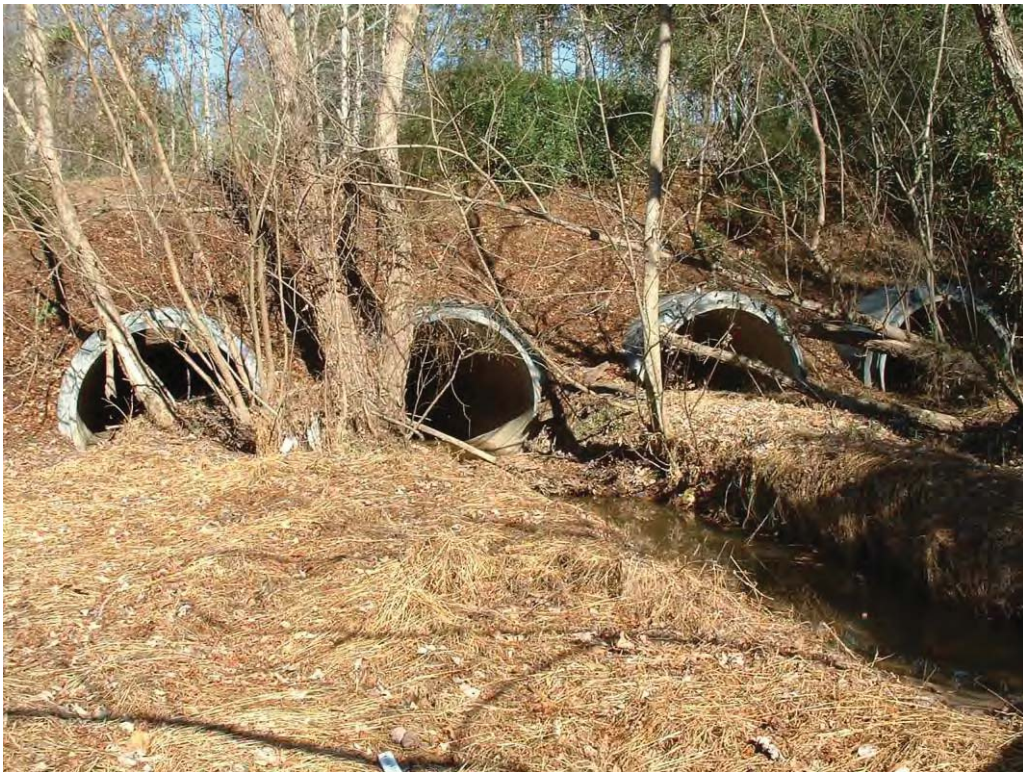
Exhibit C-3. Photos of Sedimentation at Culverts
