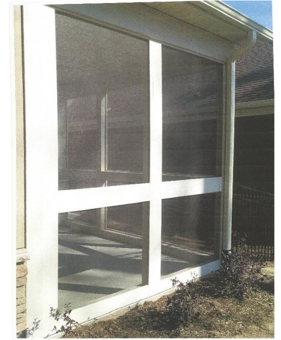
Vinyl Soffit + Al. Gutters
