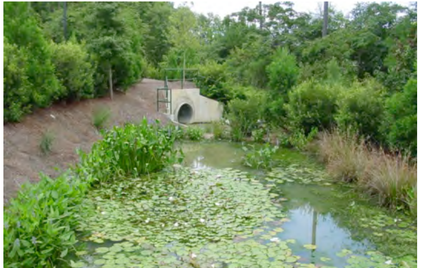
Stormwater Management: Constructed wetlands
