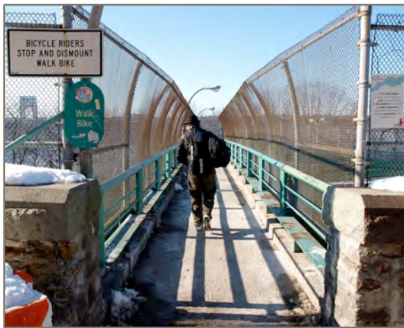
This bridge is too narrow for safe passage and aesthetically inappropriate for a gateway feature.
