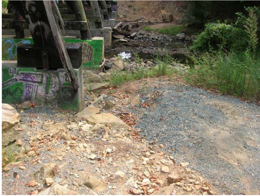
Stormwater flows past the railroad trestle footers and directly into Bolin Creek. Facing south.
