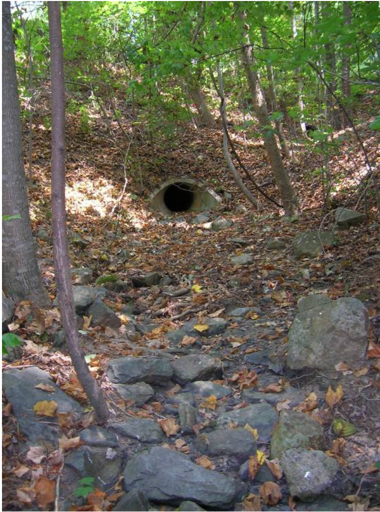
The stormwater outfall at Site 23, which flows into the existing basin. Facing north and upstream.
