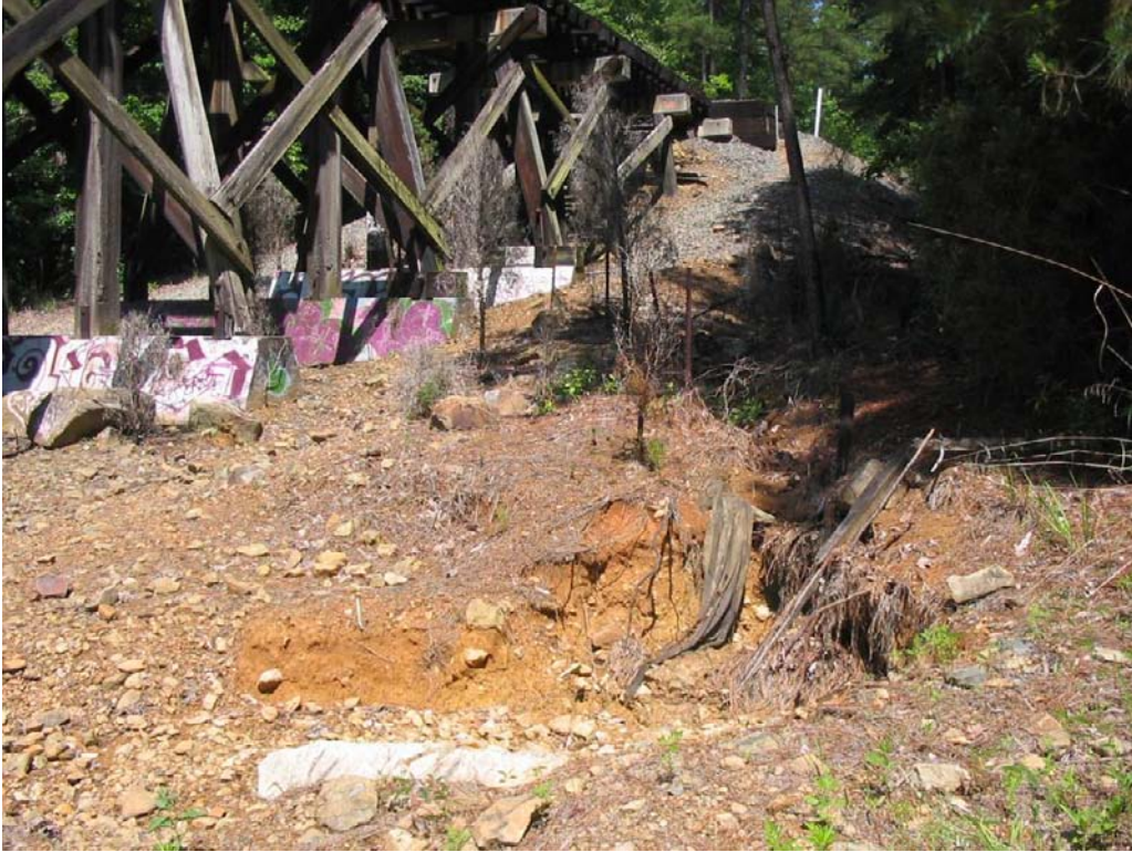
A view of the erosion occurring adjacent to a railroad trestle. Facing north.
