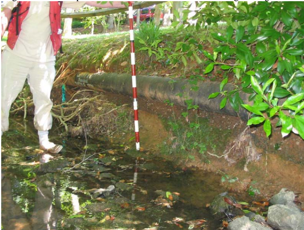
A utility line runs parallel with the streambank, just upstream of Cobblestone Drive crossing.
