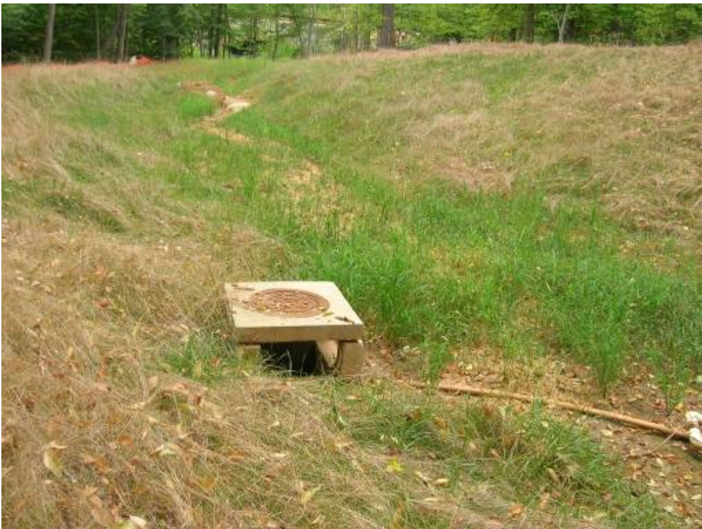
Another sediment basin at Site 6. Note the eroding grassy swale leading into the basin. Facing east.
