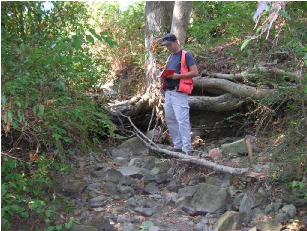
The stream is severely incised, and has degraded below the roots of several large trees. Facing upstream.
