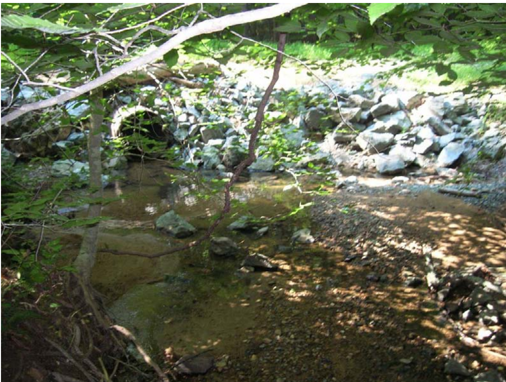
A utility crossing near Site 28 has caused mass wasting on the stream banks.
