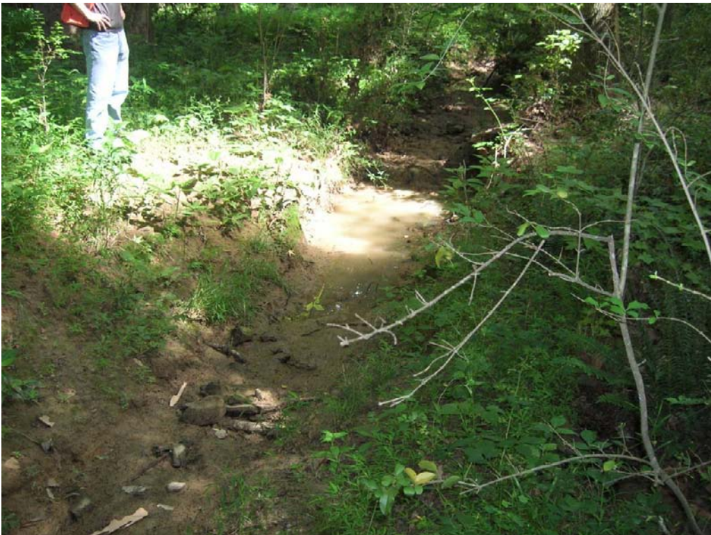
A view of a stormwater scour area flowing from the paved roads of a residential area into the floodplain ditch.
