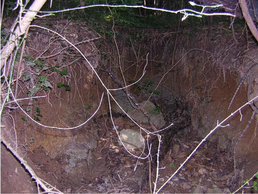
One of the headcuts present at Site 29. Looking upstream.
