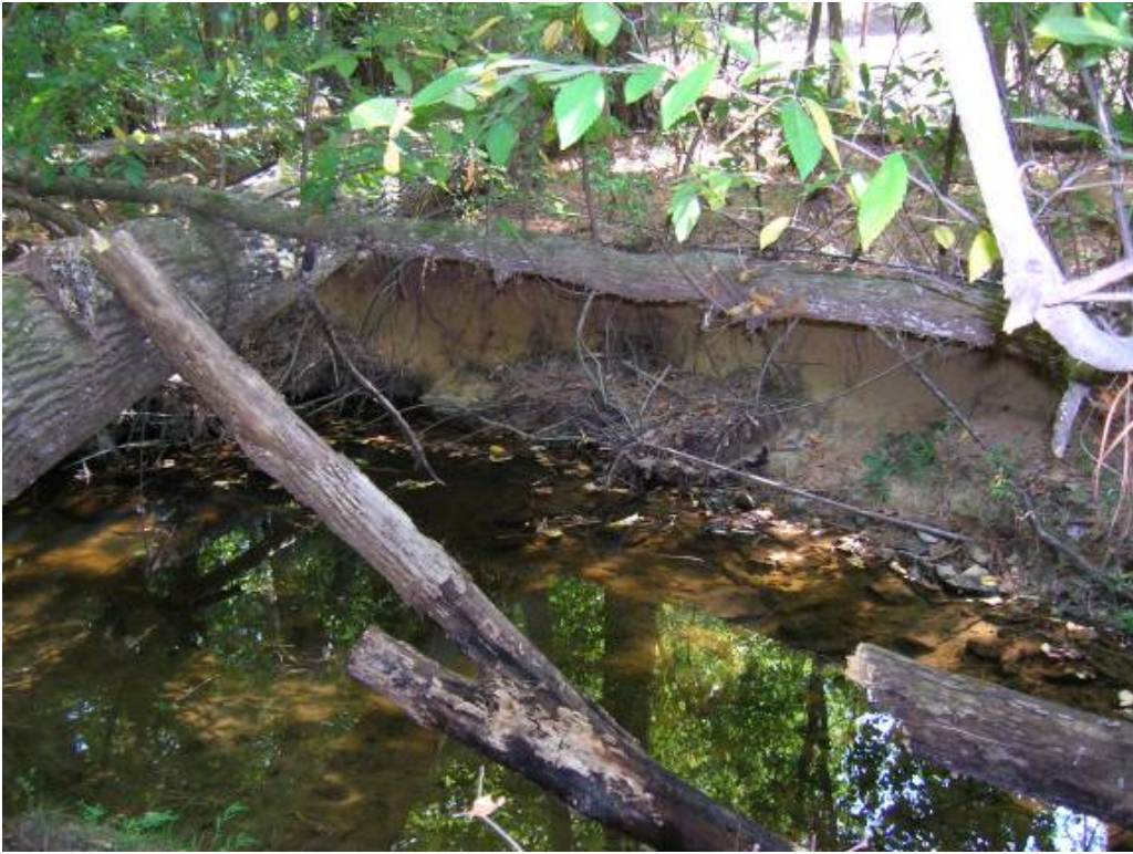
Eroding streambanks downstream of the road crossing. Facing towards right bank.
