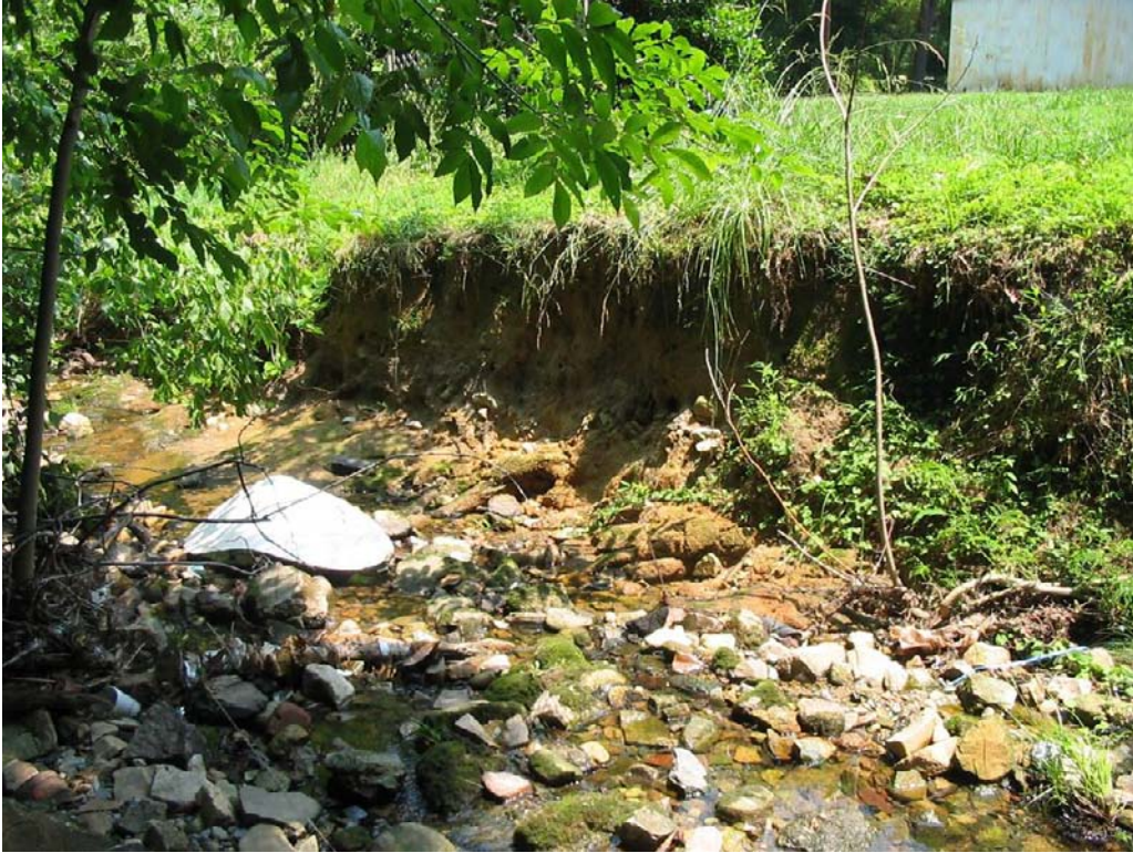
Severe bank erosion is occurring along this reach. Facing upstream.
