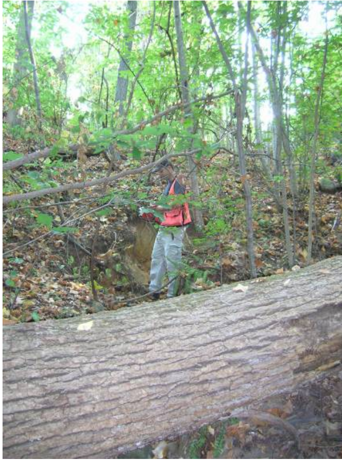
Flow from the stormwater outfall is causing hill erosion before flowing into the existing BMP. Facing northeast.
