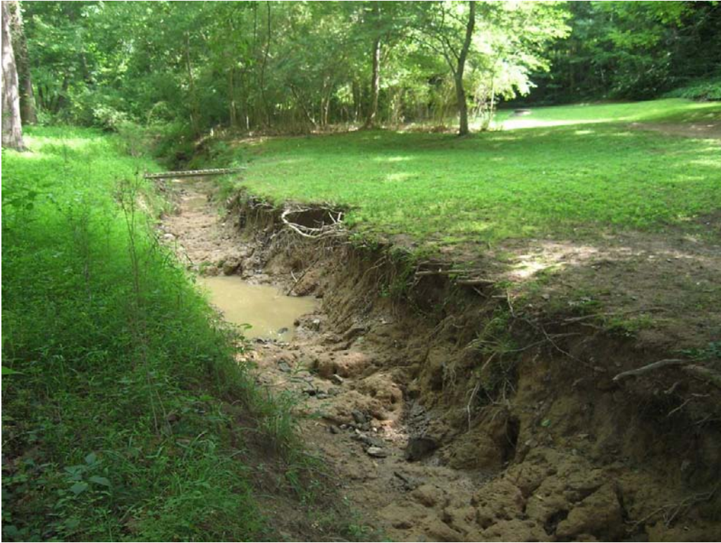
A ditch was dug in the floodplain of Battle Branch. On the right side of the photo is a residential backyard. The left side of the photo is the floodplain and utility easement along Battle Branch. Facing downstream.
