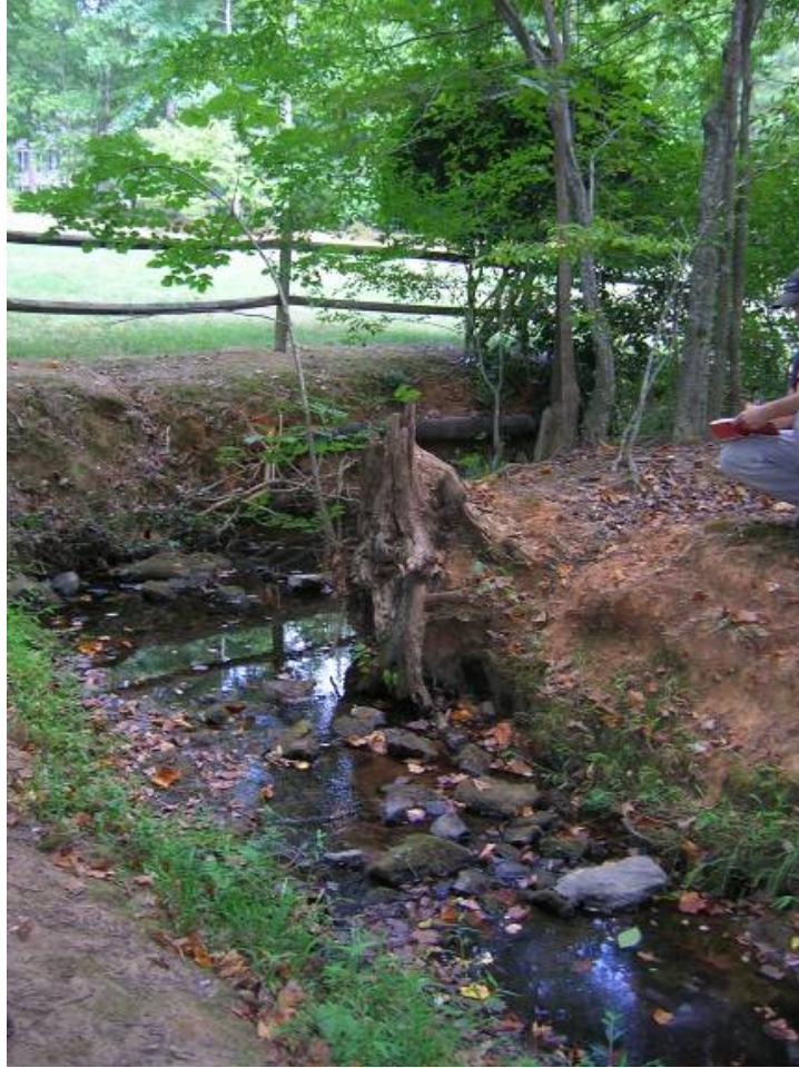
Eroding stream banks upstream of the Cobblestone Drive crossing. Facing downstream.
