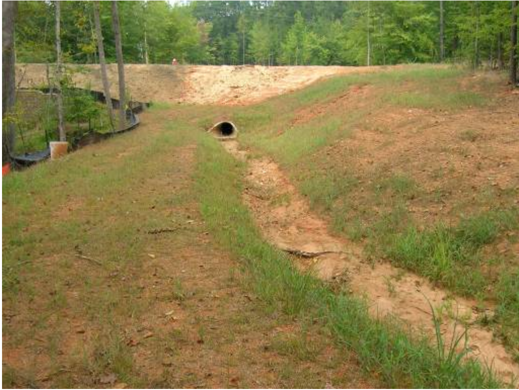
An eroding grassy swale, facing west.
