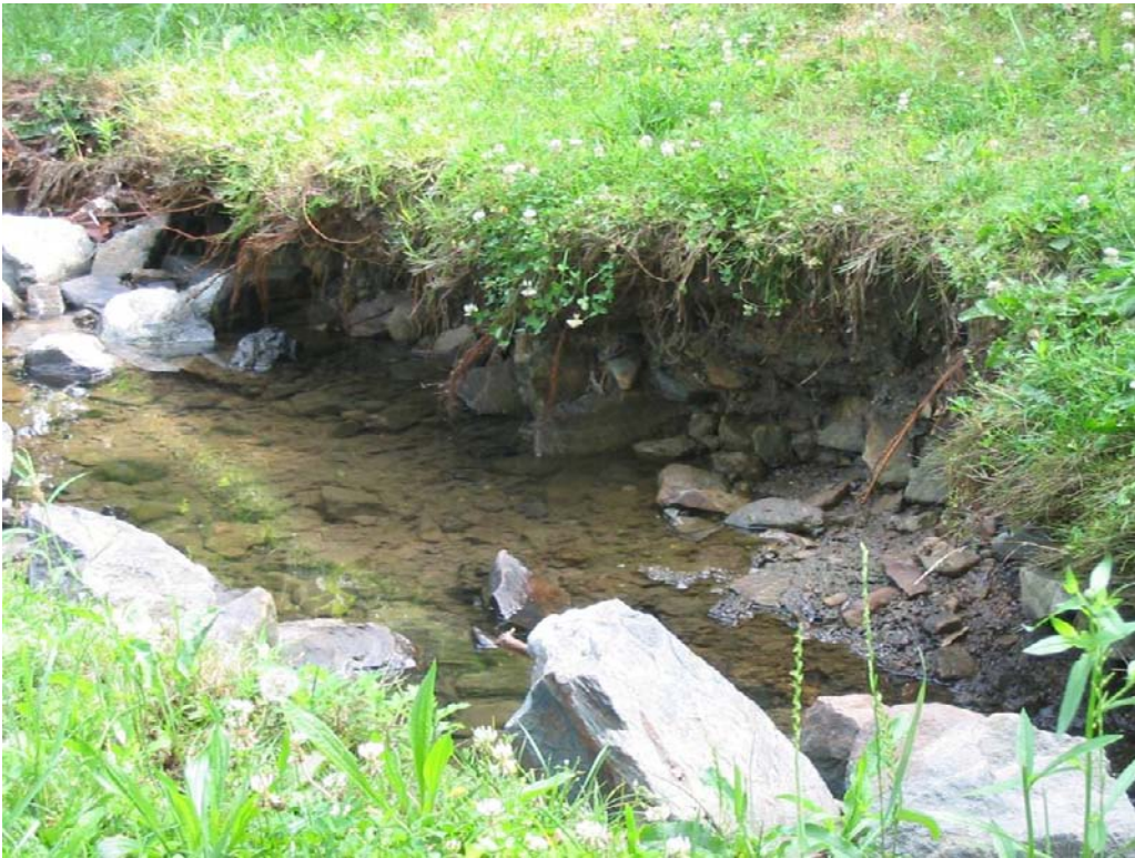
Mass wasting is occurring along this reach. Facing upstream.
