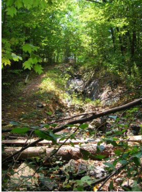
Facing uphill towards the outlet pipe that discharges into a rip-rap lined ditch.
