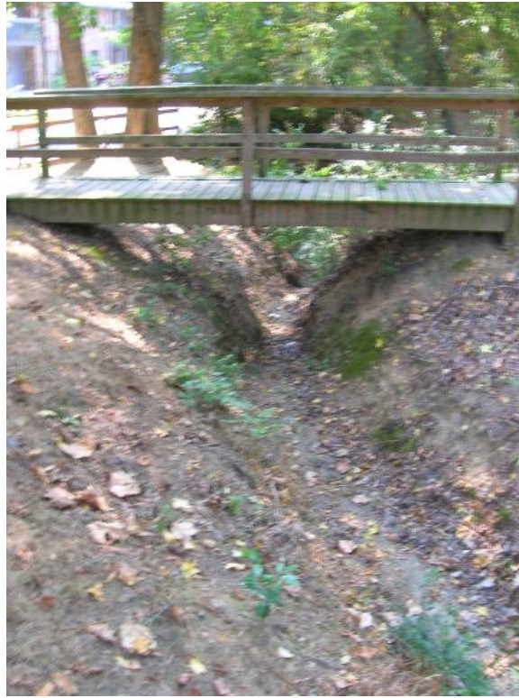
What was observed to be an ephemeral stream joins the main channel after flowing under Estes Drive Ext. Facing downstream.
