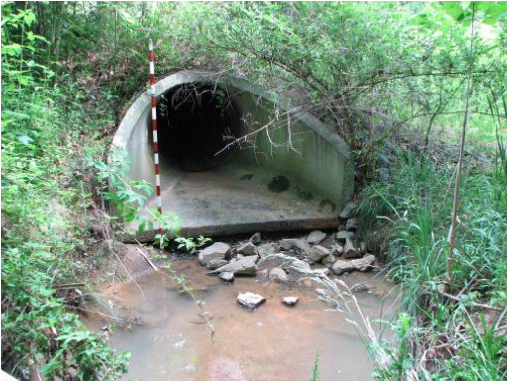
The pipe outlet discharging stormwater from the middle school. Facing south towards the middle school.
