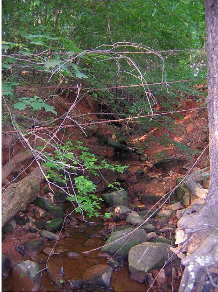
A degraded and eroding spillway on Bolin Creek just below the pond dam. Facing upstream towards the dam.
