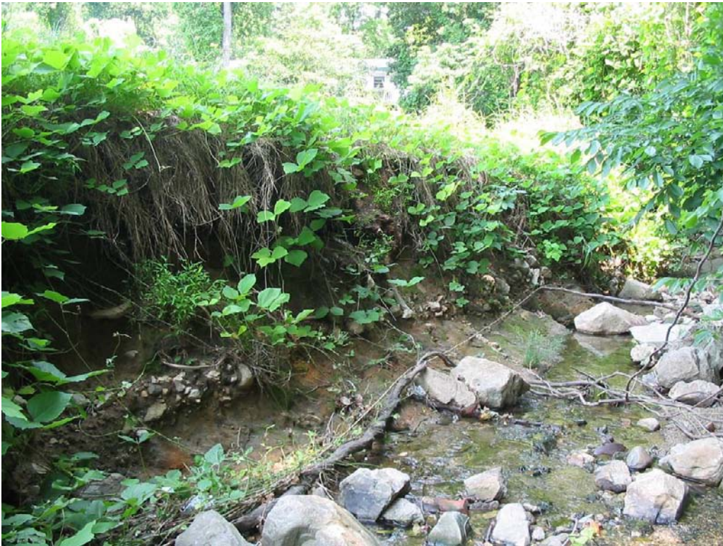
Another view of the incised channel and bank erosion. Kudzu dominates the floodplain of the stream. Facing downstream.
