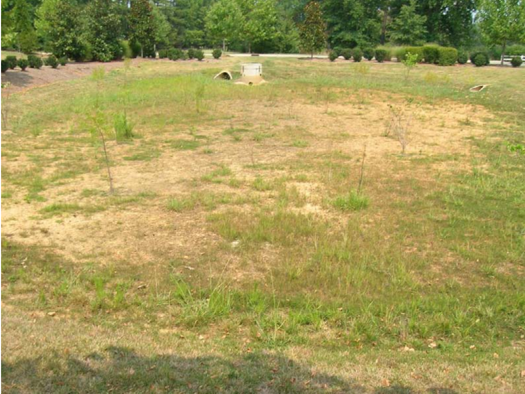
The existing stormwater basin. Note the lack of vegetation and the close proximity of the inlet pipe to the outlet structure.
