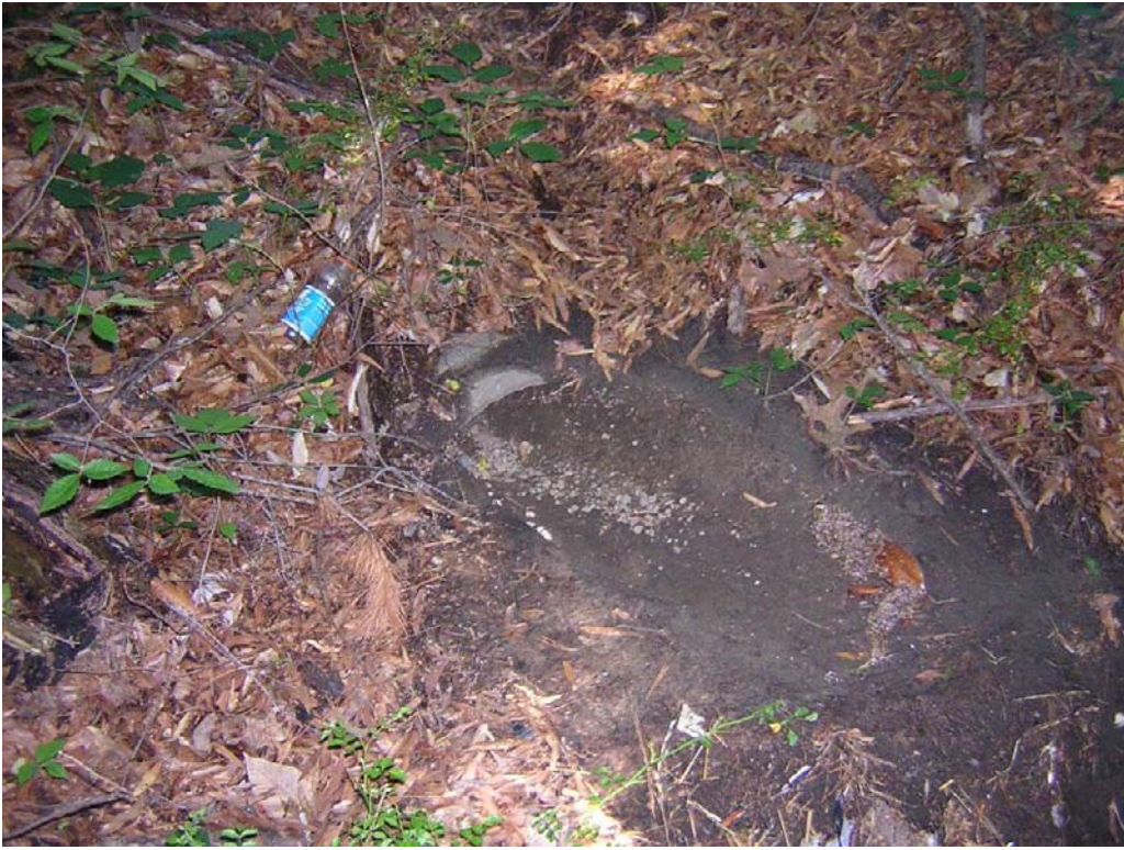
The stormwater outfall pipe from Hillsborough Street is almost completely buried. Facing northwest.
