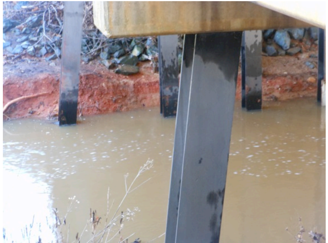
Urgent note: Erosion and water on east side of Homestead Bridge extends behind the steel bridge supports
