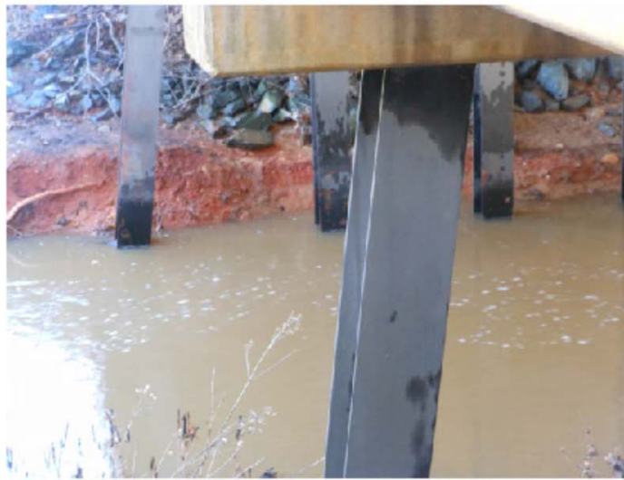
Urgent note: Erosion and water on east side of Homestead Bridge extends behind the steel bridge supports
