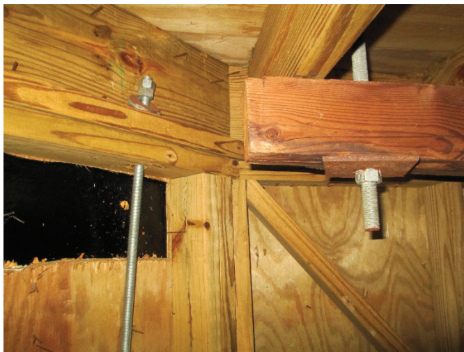
View of loose threaded rod inside the cupola.
