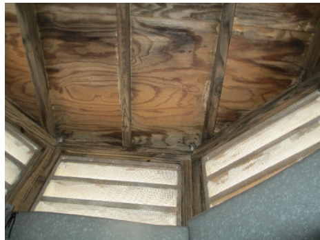
Evidence of moisture at interior of cupola. Structural damage not yet significant.
