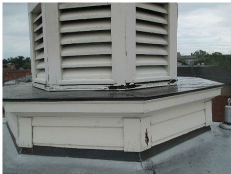
Water damage to trim of cupola.
