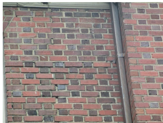
Deteriorated mortar below area in left photo.
