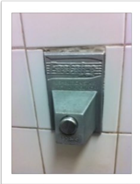
This hand dryer is less vulnerable to misuse or breakage because it is embedded in the wall.
