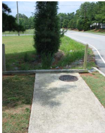
Summer 2004, sidewalk ends abruptly outside Legion Post, Legion Road. A sidewalk extension is scheduled for construction 2005.
