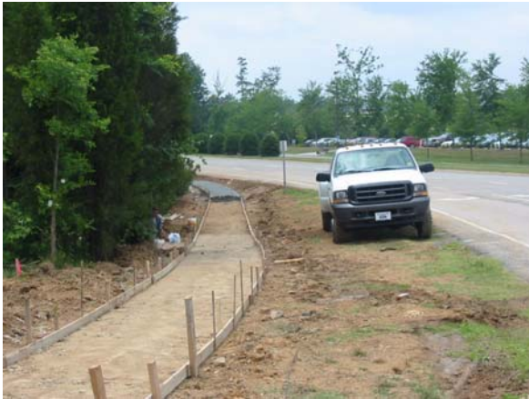
Summer 2004, sidewalk under construction along Friday Center Drive. Required as part of the development of the Marriott Hotel off NC 54
