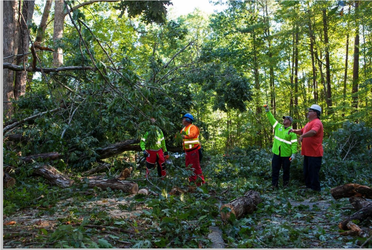
Public Works crew managing debris after a major storm
