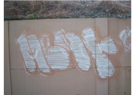
Vandalism – Please report it! This tagging along the Bolin Creek Trail has been removed
