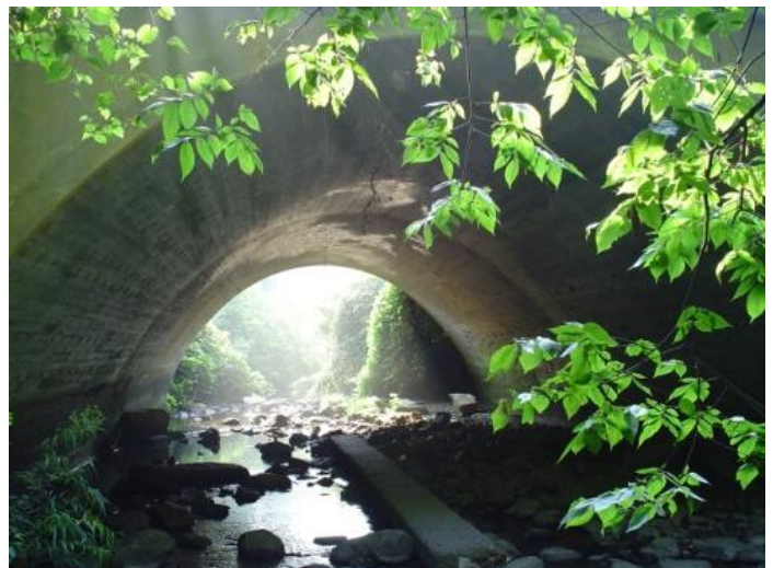
View beneath Martin Luther King Jr. Blvd. – Future route of the Bolin Creek Trail, Phase 3
