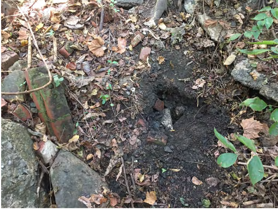
Photograph 5: Example of brick and concrete debris observed on the embankment.
